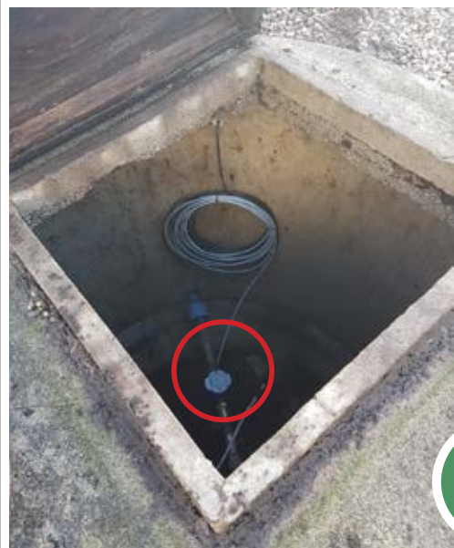
The external antenna mounted on the meter in pit. The cable has a proper length.
