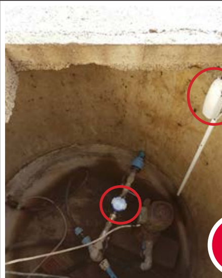
Meter with pit antenna. The antenna is mounted under the pit cover which does not result in better signal conditions.
