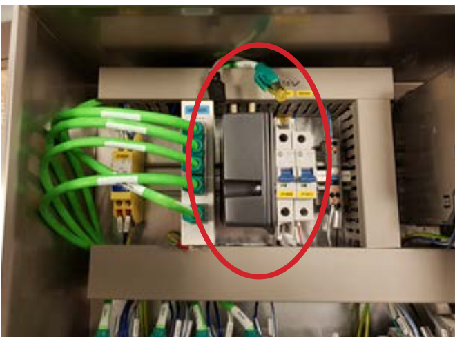
Figure 37 - SIERRA Wireless RV50x Installation
