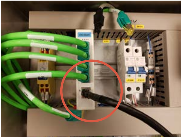
Figure 34 - READy Collector Base LAN connection
